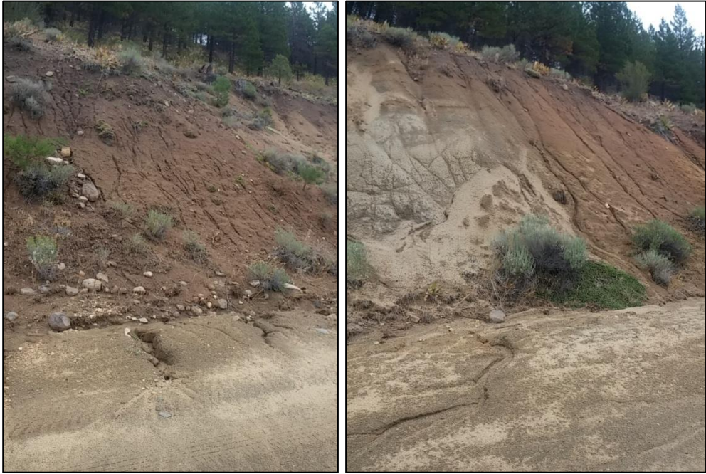
Figure 8. Cutslope rills and road surface gullies that increased and expanded during summer thunderstorms.
