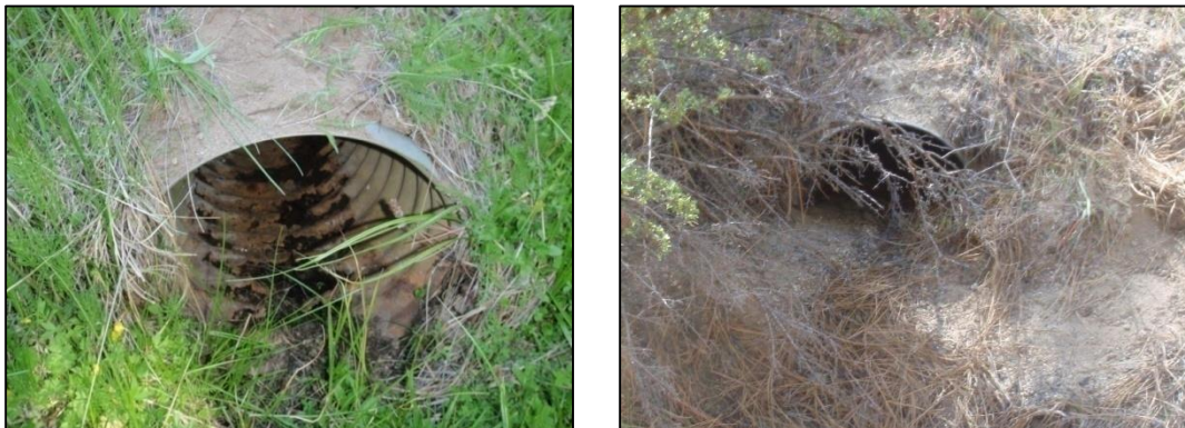
Figure 36. Problems with ditch relief culverts. The left culvert is rusted through. The right culvert has an occluded inlet.
