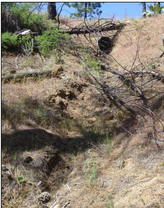
Figure 27. Gully below the outlet of a ditch relief culvert.
